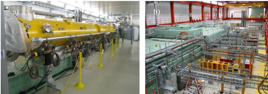
Figure 2: Photographs of an installed cryomodule (left) and the shielded tunnel and installed rf and power supply infrastructure (right).
