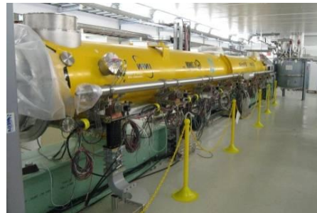
Fig. 10: The first cryomodule from DESY installed in the ASTA facility at Fermilab. This has eight 9-cell cavities.
